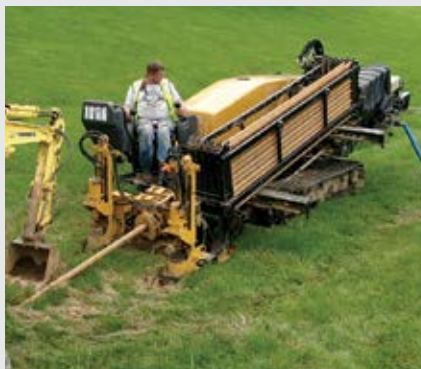
Installation of the fiber line for the GATEway Fiber Network, which spans over 19 miles
